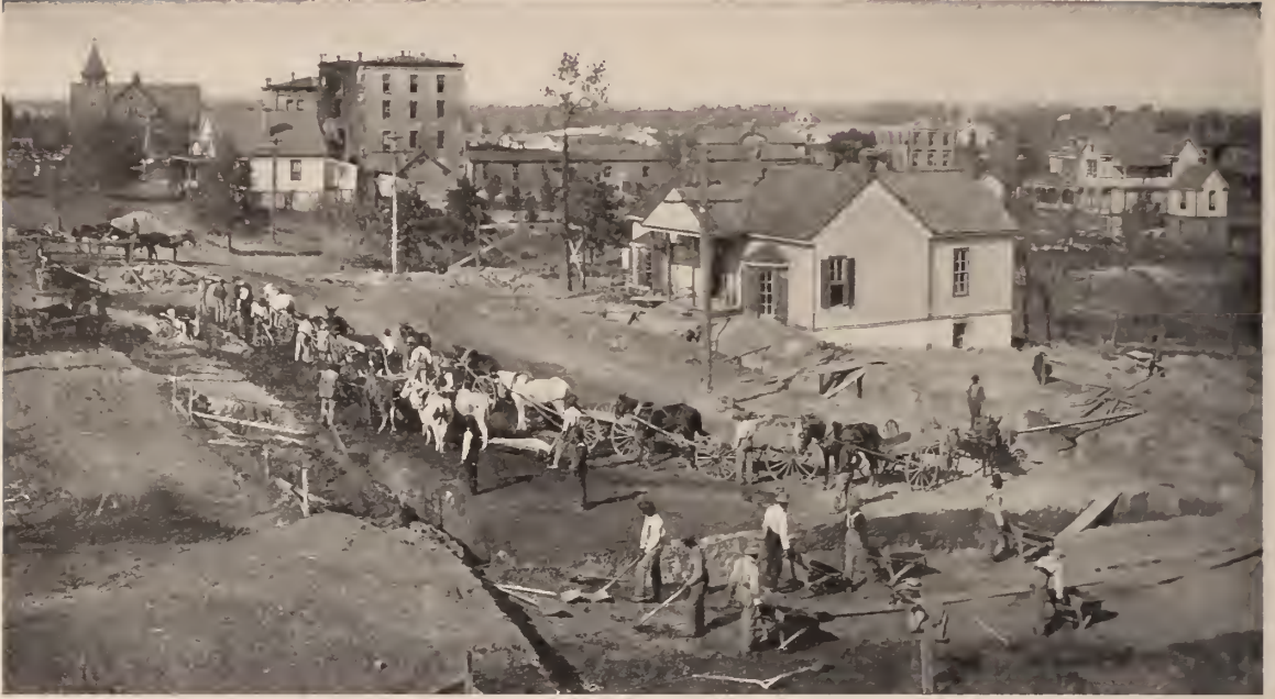
THE STUDENTS DIGGING THE FOUNDATIONS FOR THE C. P. HUNTINGTON MEMORIAL BUILDING
